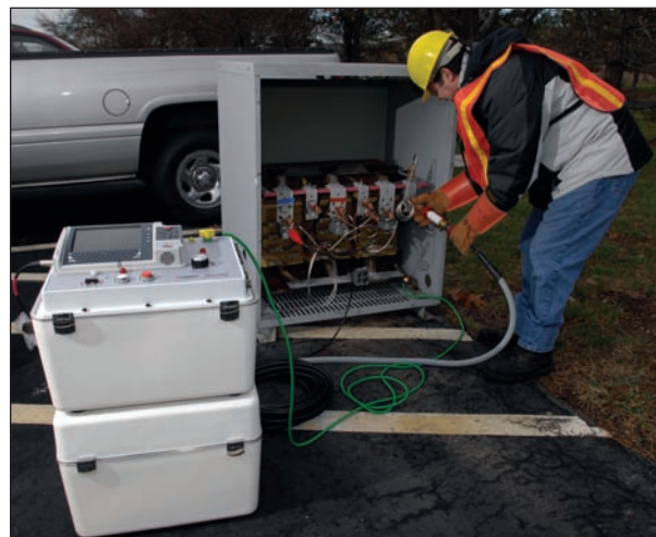
DELTA3000 shown testing a pad mount transformer
