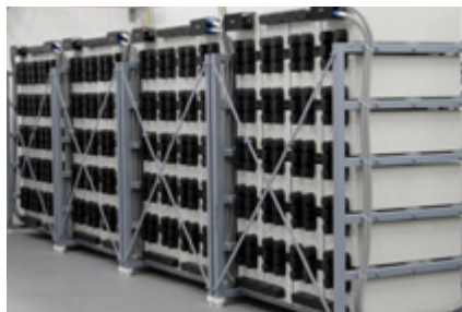
Energy Storage System
